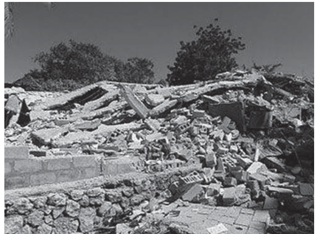
The remains of the CONASPEH building.
